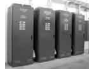
Power Master Installed
